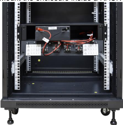
Fig. 2. Mounting of the controller in a RACK cabinet.
